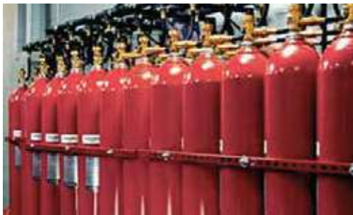
GAS SUPPRESSION & VALVES
