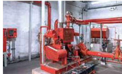
FIRE PIPING, PUMP
